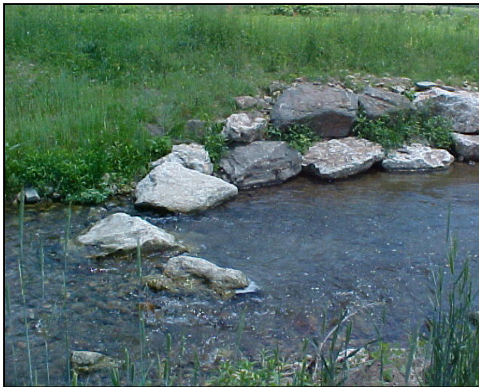
In-stream structures such as this J-hook can be installed to minimize erosion of the newly restored streambank until vegetation becomes established.
