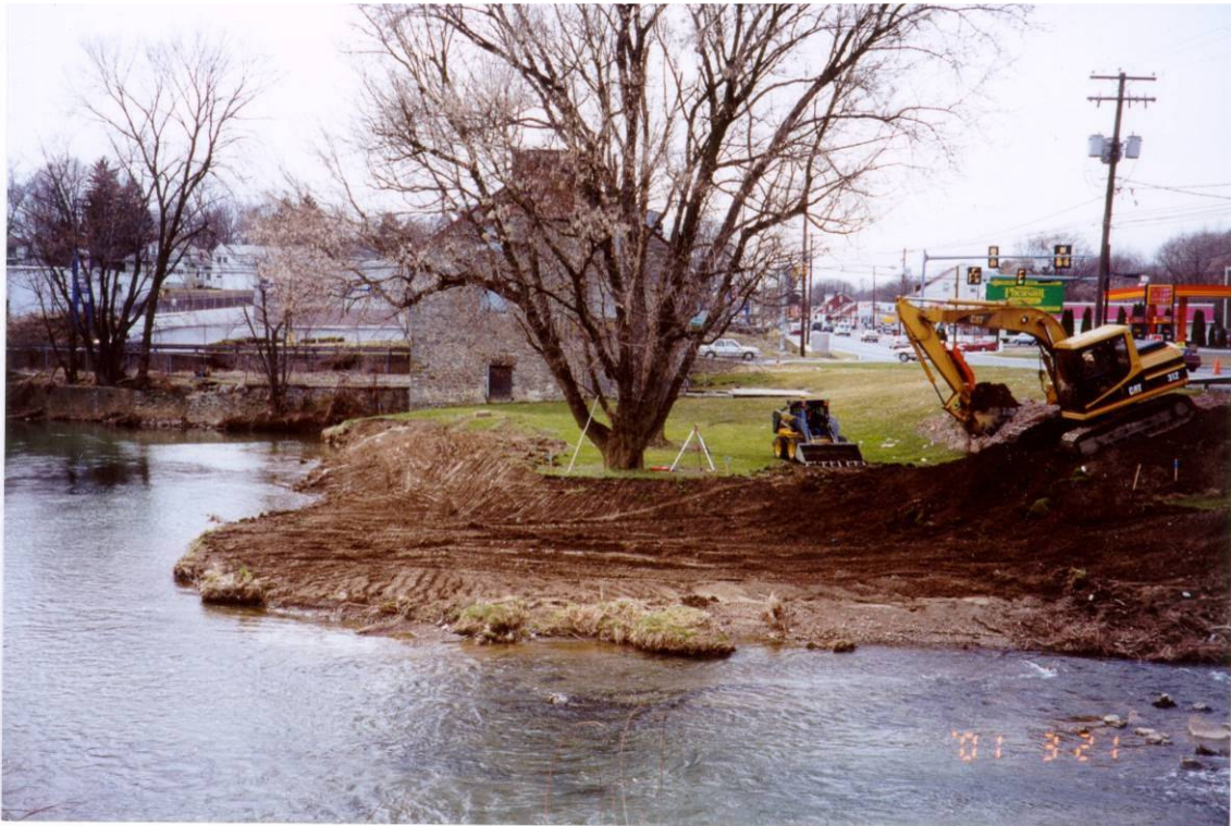
Sample photograph of floodplain restoration – removing previously placed fill and legacy sediments
